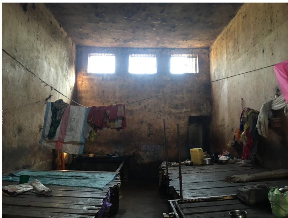
One of the cells shared by more than 40 detainees in MC Maintirano. Mold is visible on the walls and the wooden planks are rotting. August 2017 @ Amnesty International
